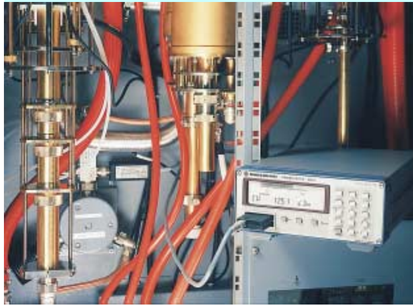
NRVS in use: on-site measurement on TV transmitter
